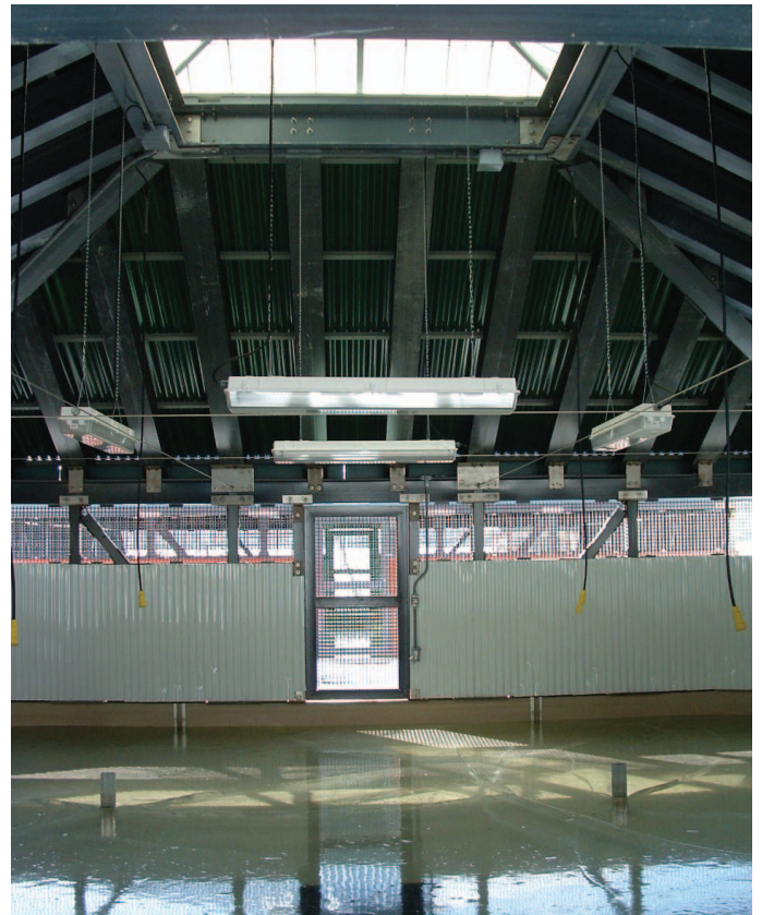
The Craig Brook National Fish Hatchery in East Orland, Maine used corrosion resistant EXTREN® structural shapes to frame roofing structures over moisture rich crowding pools.
