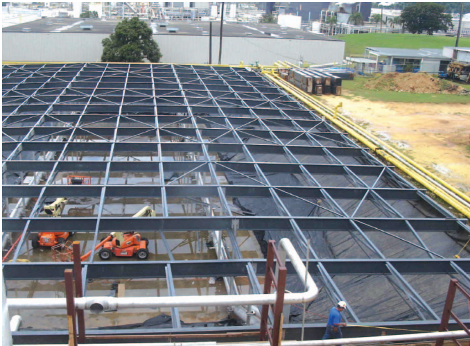
An odor control cover was constructed using EXTREN® structural shapes for a waste water treatment facility in Puerto Rico.
